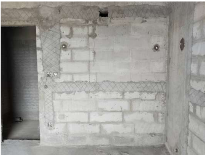
WC Electrical - Seventh Floor
