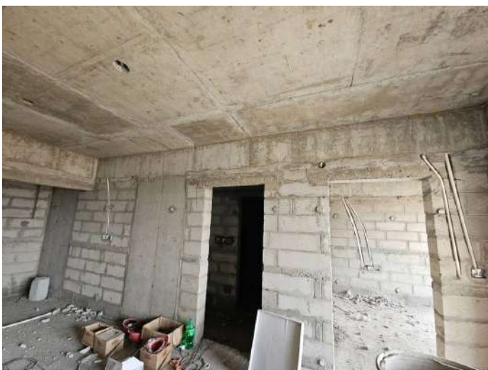
WC Electrical - Seventh Floor
