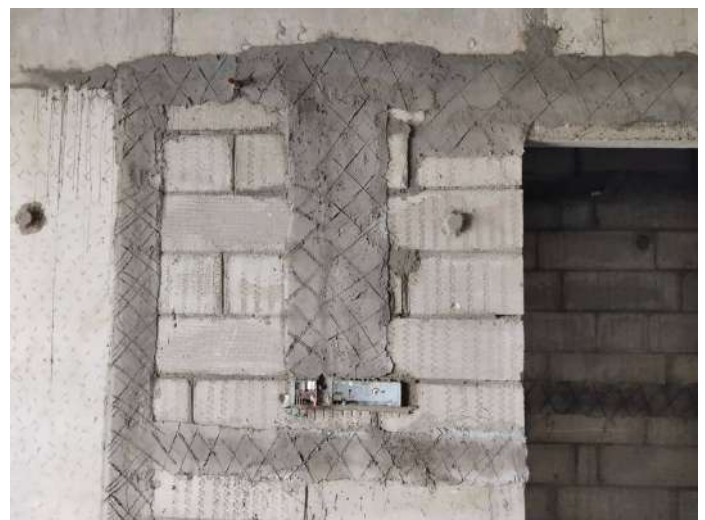
WC Electrical - Seventh Floor
