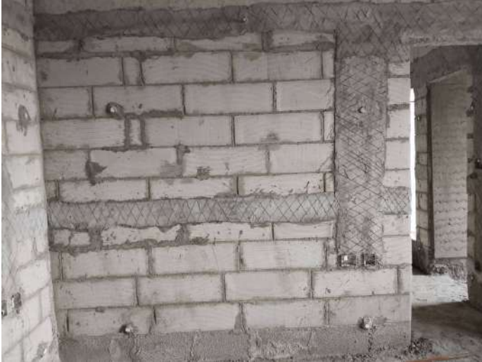
WC Electrical - Seventh Floor
