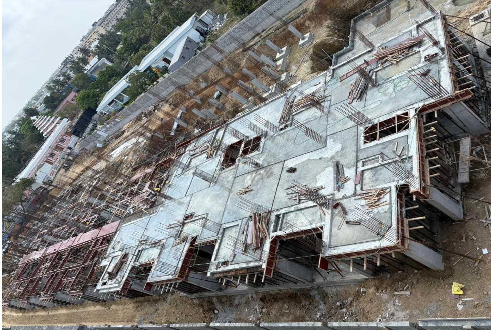
Block-4- Pour 1-First floor Slab Concrete Work Completed & Pour-2 Shuttering work in Progress
