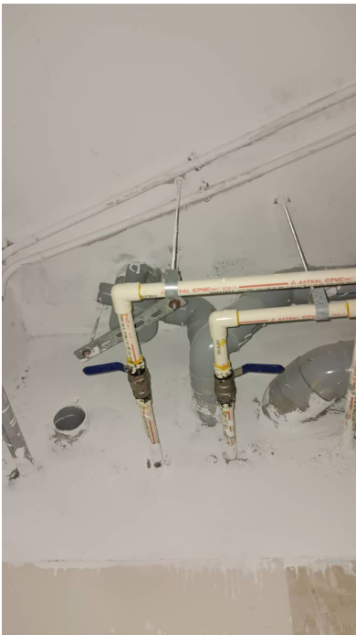
Block 4 - External Plumbing Shaft Riser to Internal
