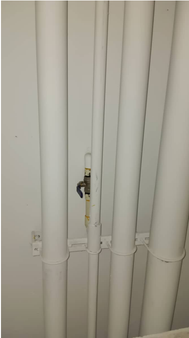
Block 4 - External Plumbing Shaft Riser to Internal
