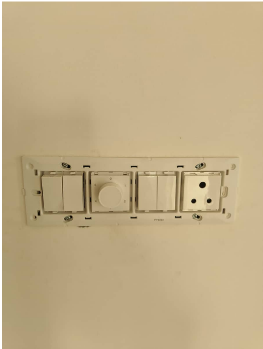
Block 4 - Switches & Socket Second Floor
