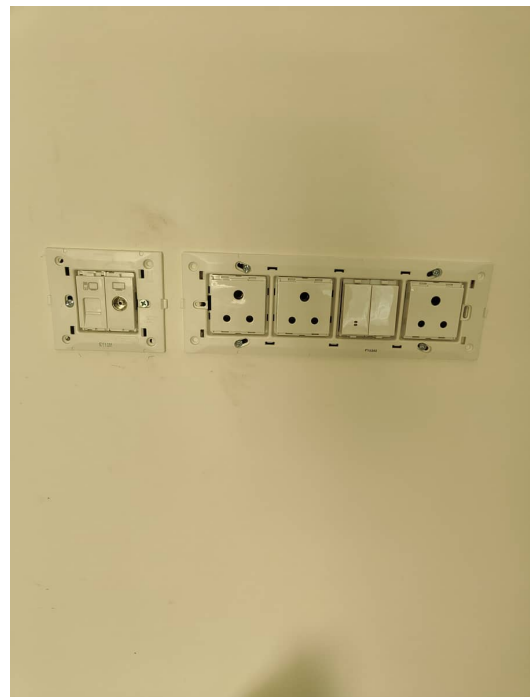
Block 4 - Switches & Socket First Floor
