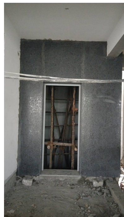
Block 4 - Lift Facia - Granite / TILE
