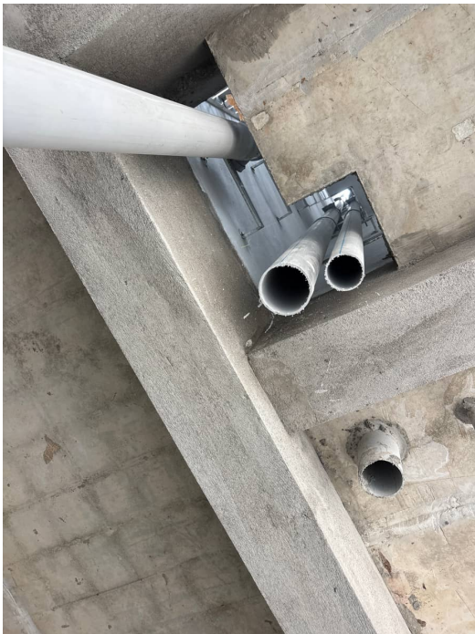
Block 2 - External Plumbing Shaft Risers
