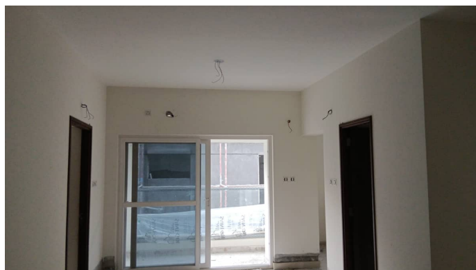
Block 4 - Switches & Socket Third Floor
