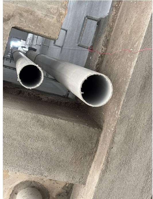
Block 2 - External Plumbing Shaft Risers
