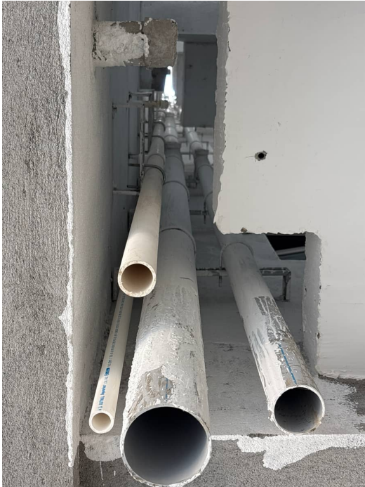
Block 2 - External Plumbing Shaft Risers
