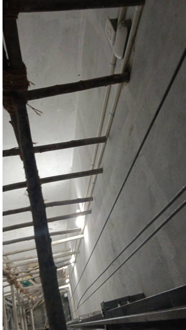
Block 4 - Elevator Electrical
