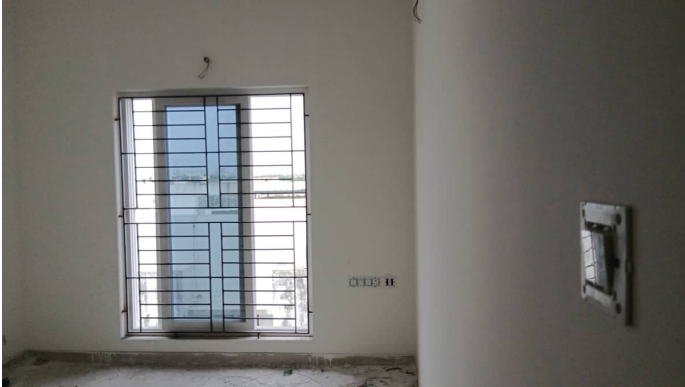
Block 4 - Switches & Socket Fifth Floor
