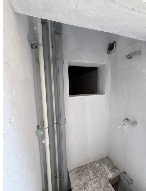
Block 2 - External Plumbing Shaft Riser to Internal
