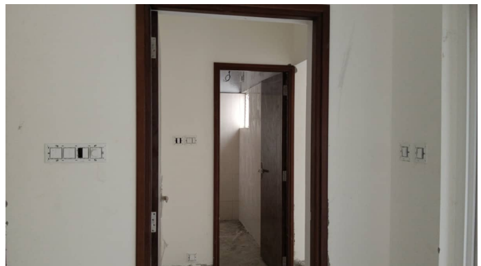
Block 4 - Switches & Socket Fourth Floor
