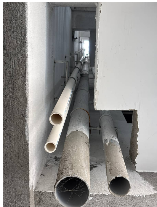
Block 2 - External Plumbing Shaft Risers
