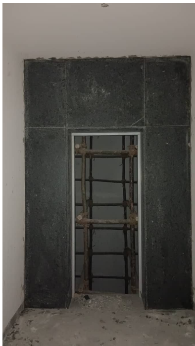
Block 4 - Lift Facia - Granite / TILE
