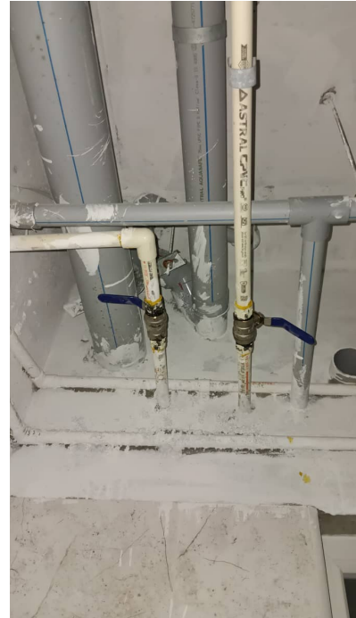
Block 4 - External Plumbing Shaft Riser to Internal
