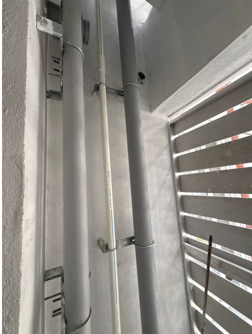
Block 2 - External Plumbing Shaft Riser to Internal
