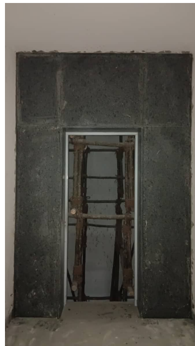
Block 4 - Lift Facia - Granite / TILE
