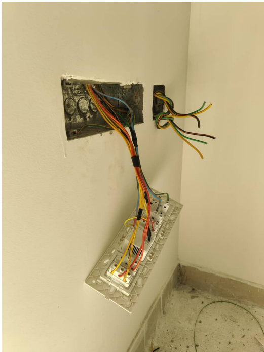
Block 4 - Switches & Socket Third Floor
