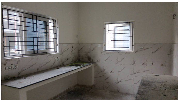
Block 4 - Switches & Socket Third Floor
