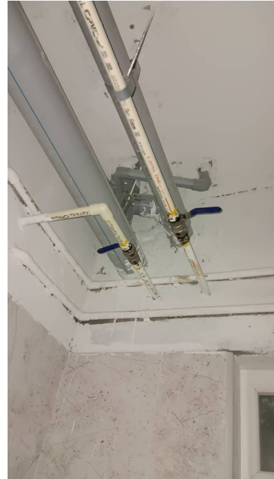
Block 4 - External Plumbing Shaft Riser to Internal
