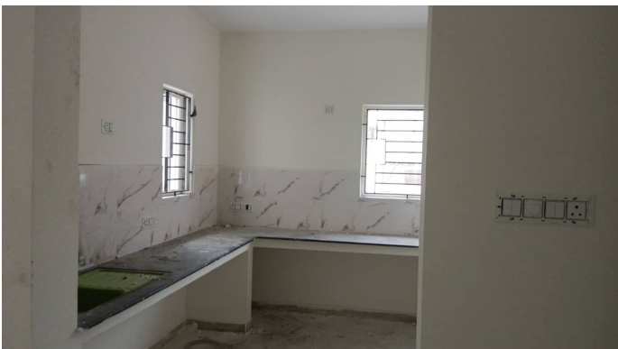
Block 4 - Switches & Socket Fourth Floor
