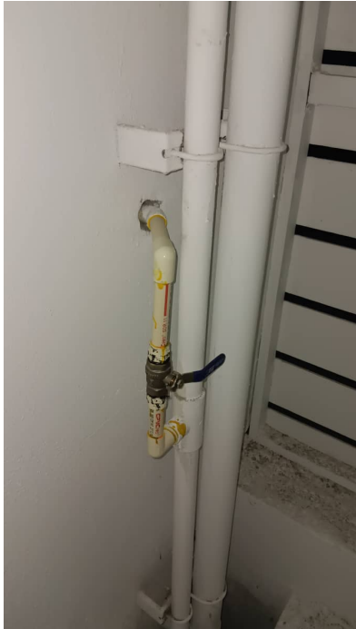
Block 4 - External Plumbing Shaft Riser to Internal
