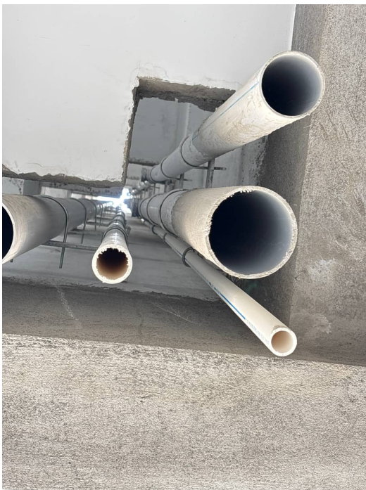
Block 2 - External Plumbing Shaft Risers
