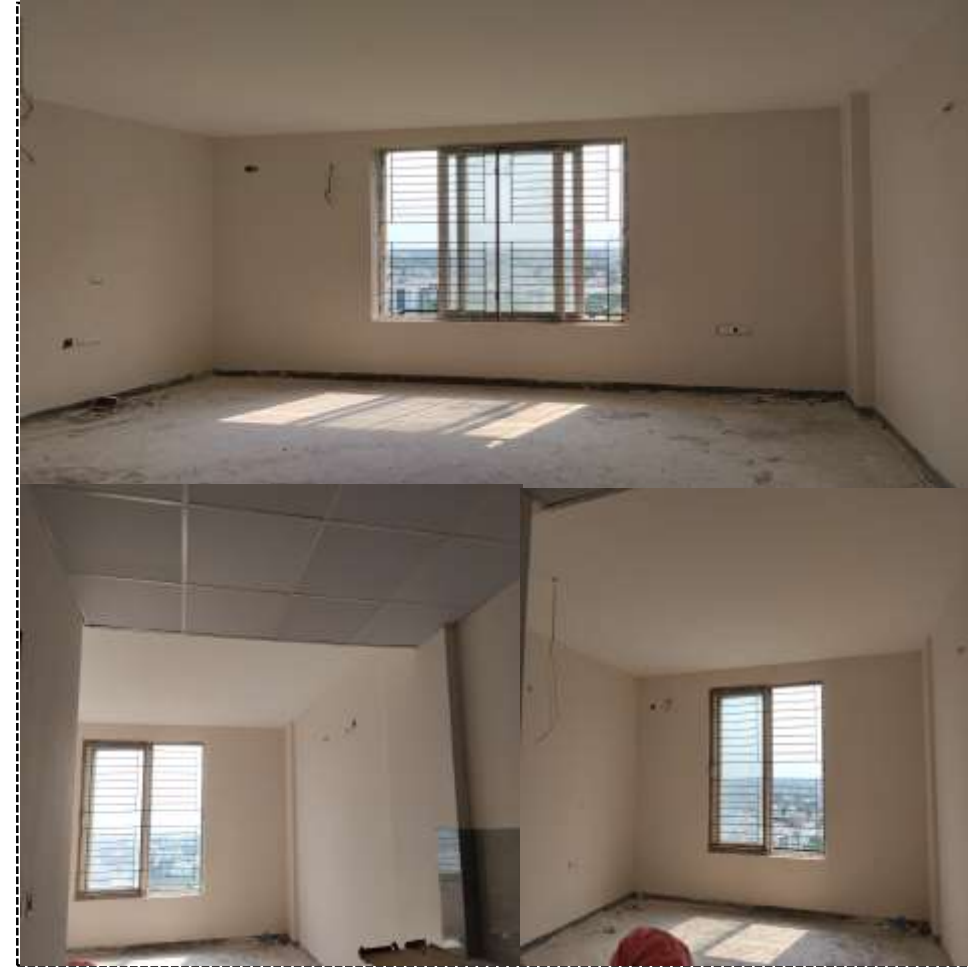
12 th & 11 th floor Ceiling & Wall 1 st Coat Painting Work Completed 10 th floor work in progress
