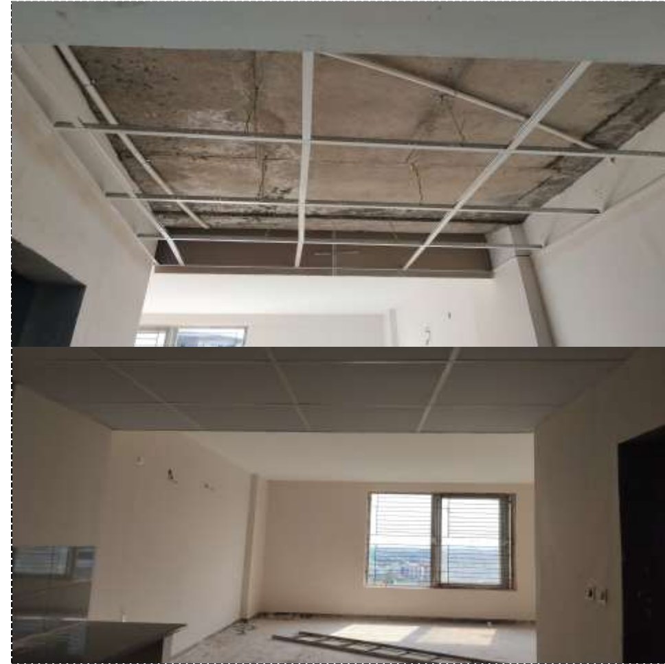
10 th floor Toilet and Kitchen Ceiling Grid False Ceiling work in Progress
