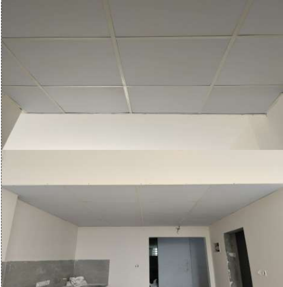
12 th & 11 th floor Toilet and Kitchen area Ceiling Grid false Ceiling work Completed
