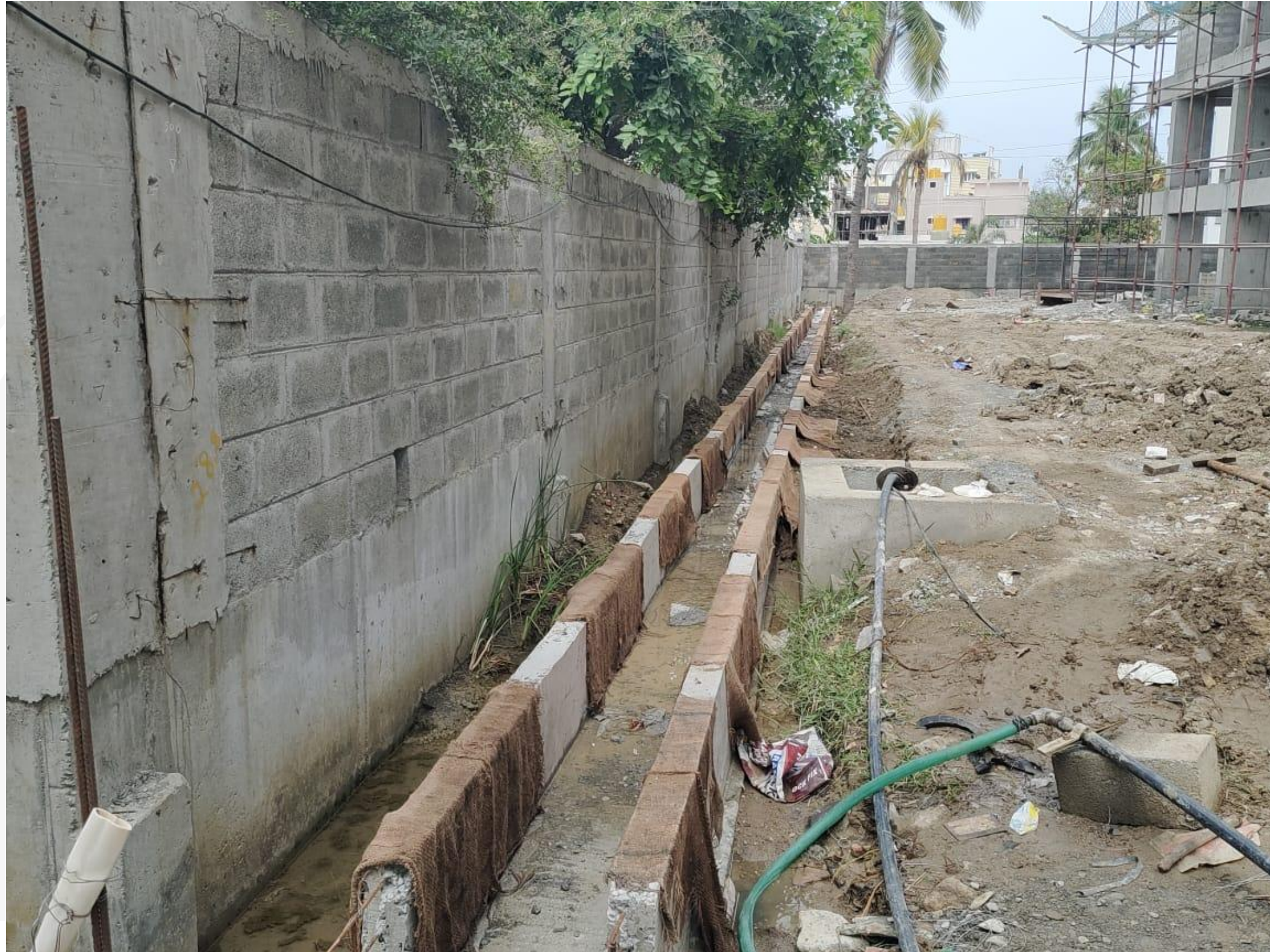
Storm Water Trench – North Side Trench Raft concrete work Completed & Wall Concrete Work In Progress.
