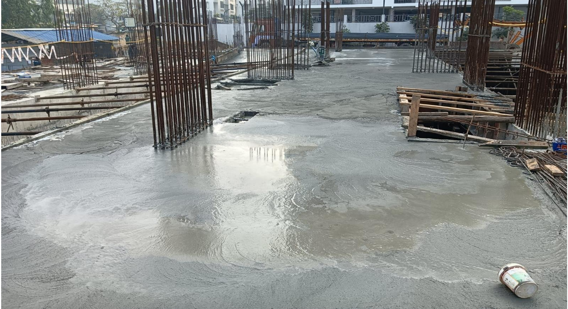
Pour-2 Basement STP cover slab and ramp area roof slab concrete work completed.
