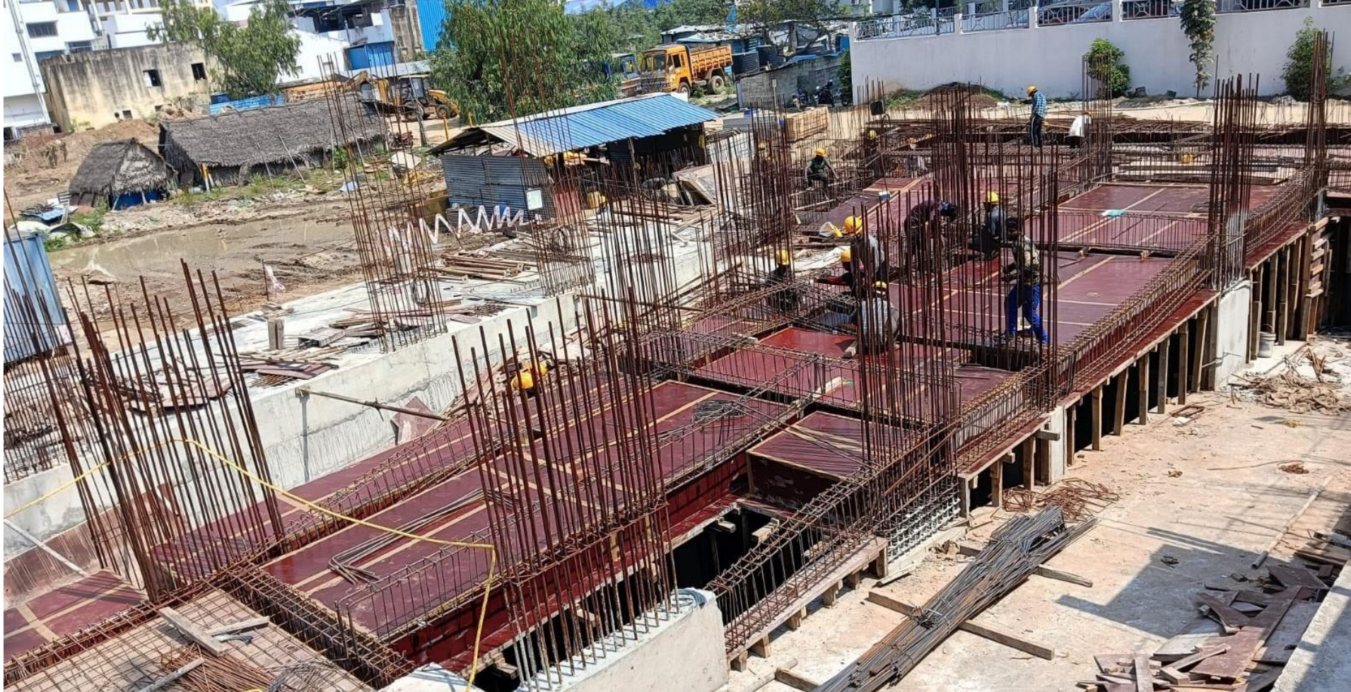
Pour-2 Basement STP cove slab and ramp area roof slab shuttering completed.
