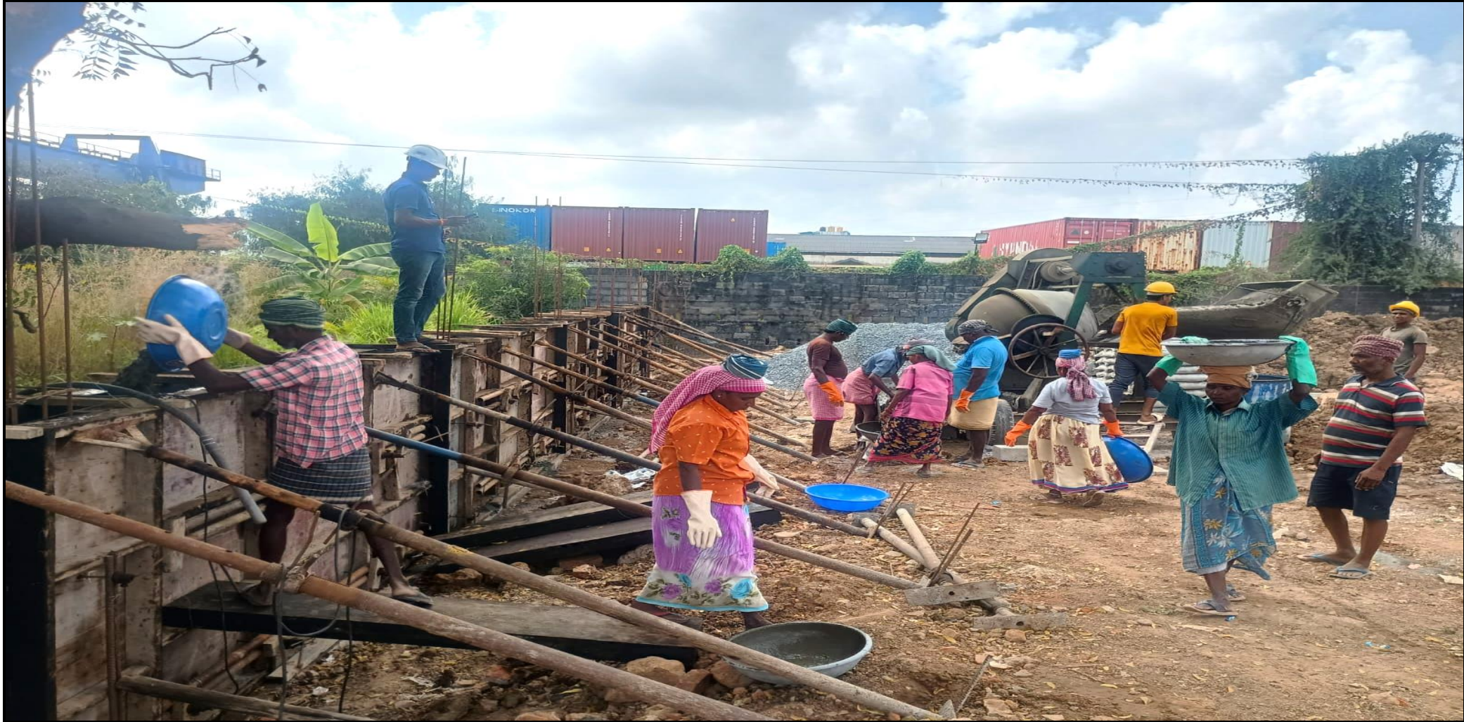
Compound wall – Plinth beam & RC wall concrete work in progress (24/113m completed)
