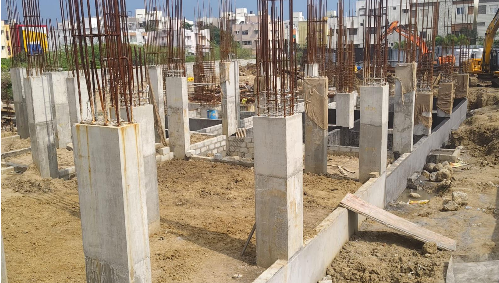
Main Building Stilt Floor Pour-1 Column 2 nd Lift Concrete Work Nearing Completion.
