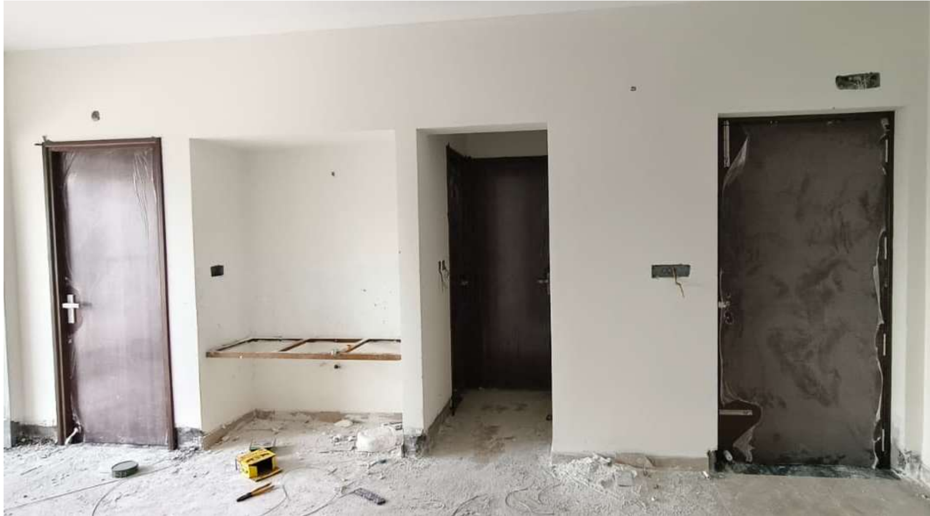
Main Building Pour-1 UP To 5 th Floor Flat Door Fixing Work Completed.
