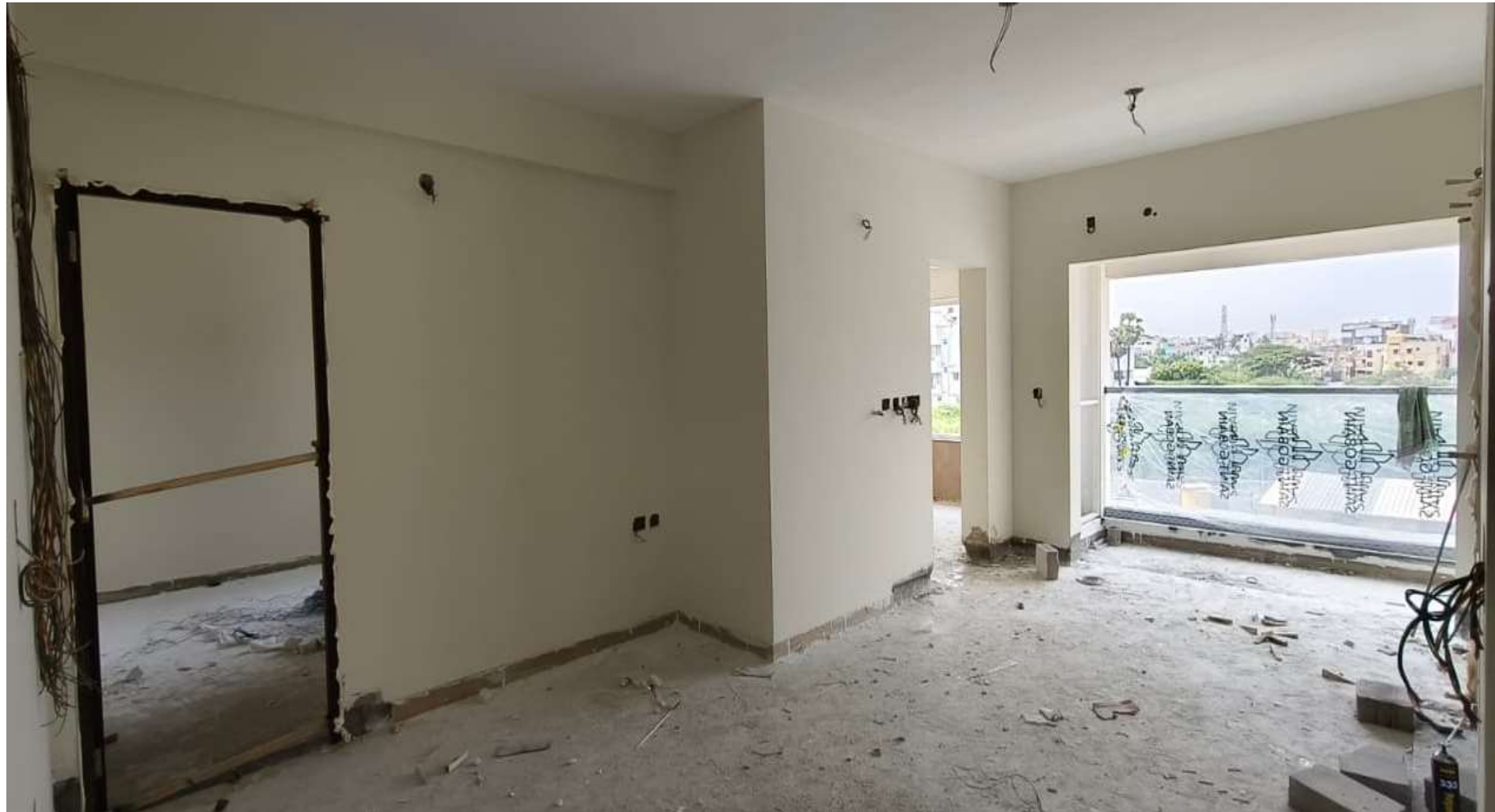
Main Building Pour-2 Electrical Up to 4 th Floor Flat Wiring Work In Progress.
