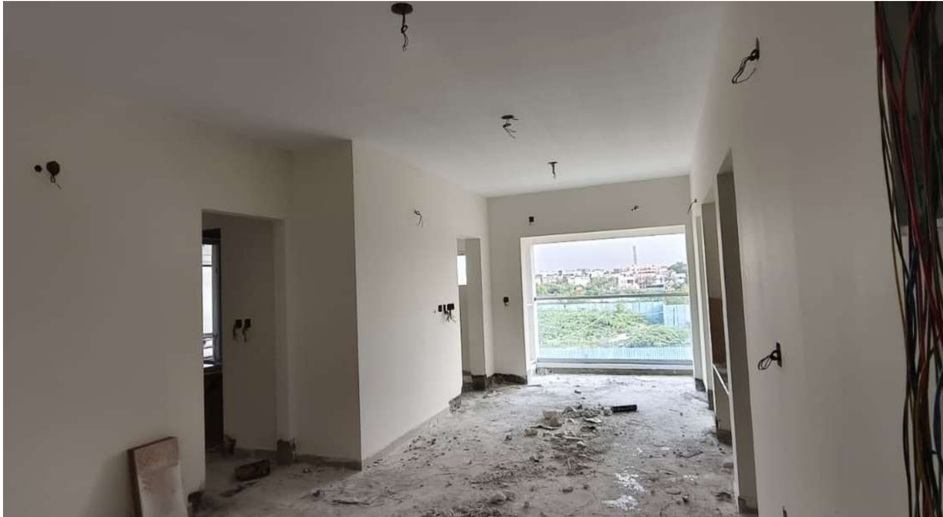
Main Building Pour-1 Electrical Up to 5 th Floor Flat Wiring Work In Progress.
