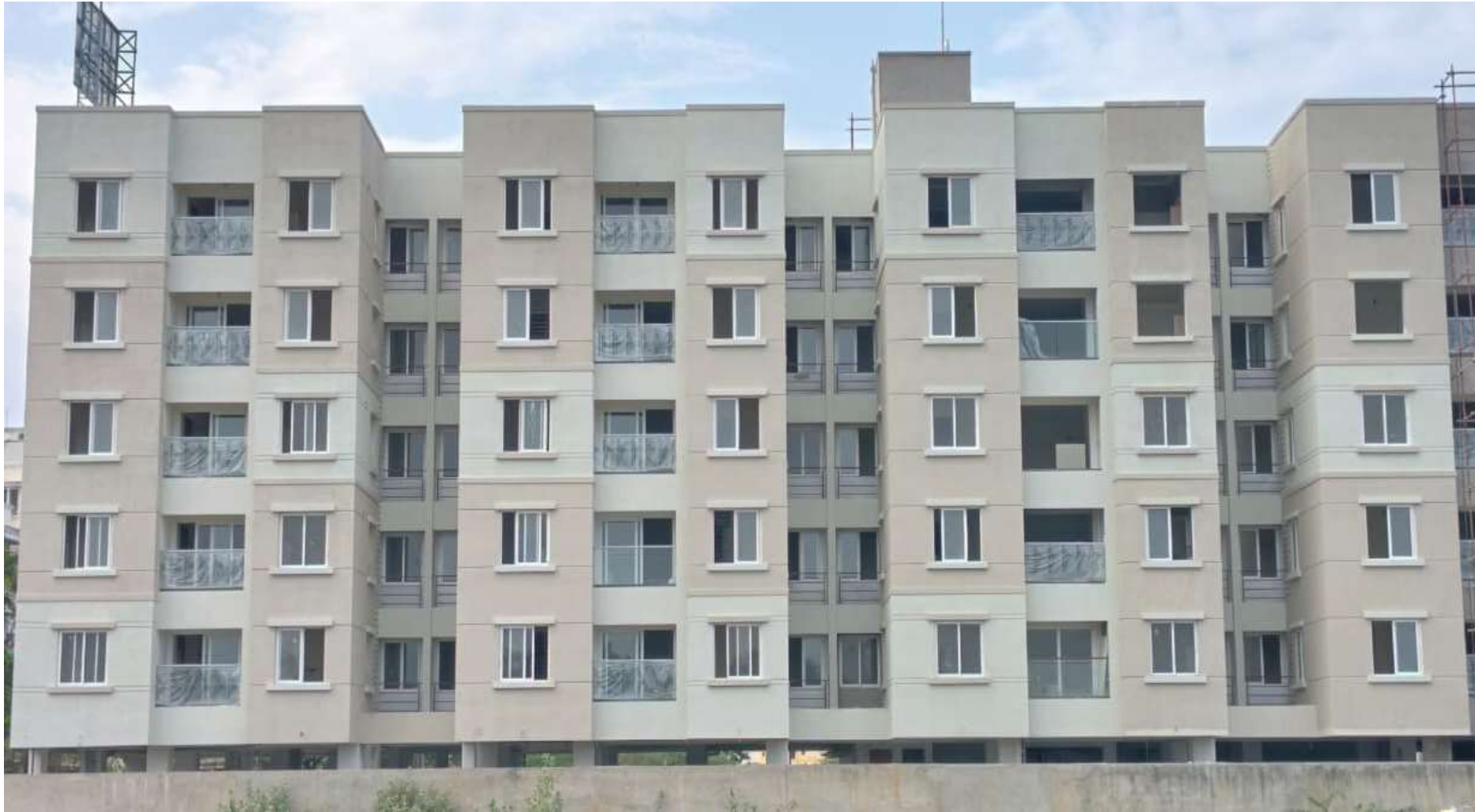
Main Building South Side External Texture Painting 1 st Coat Work In Progress.
