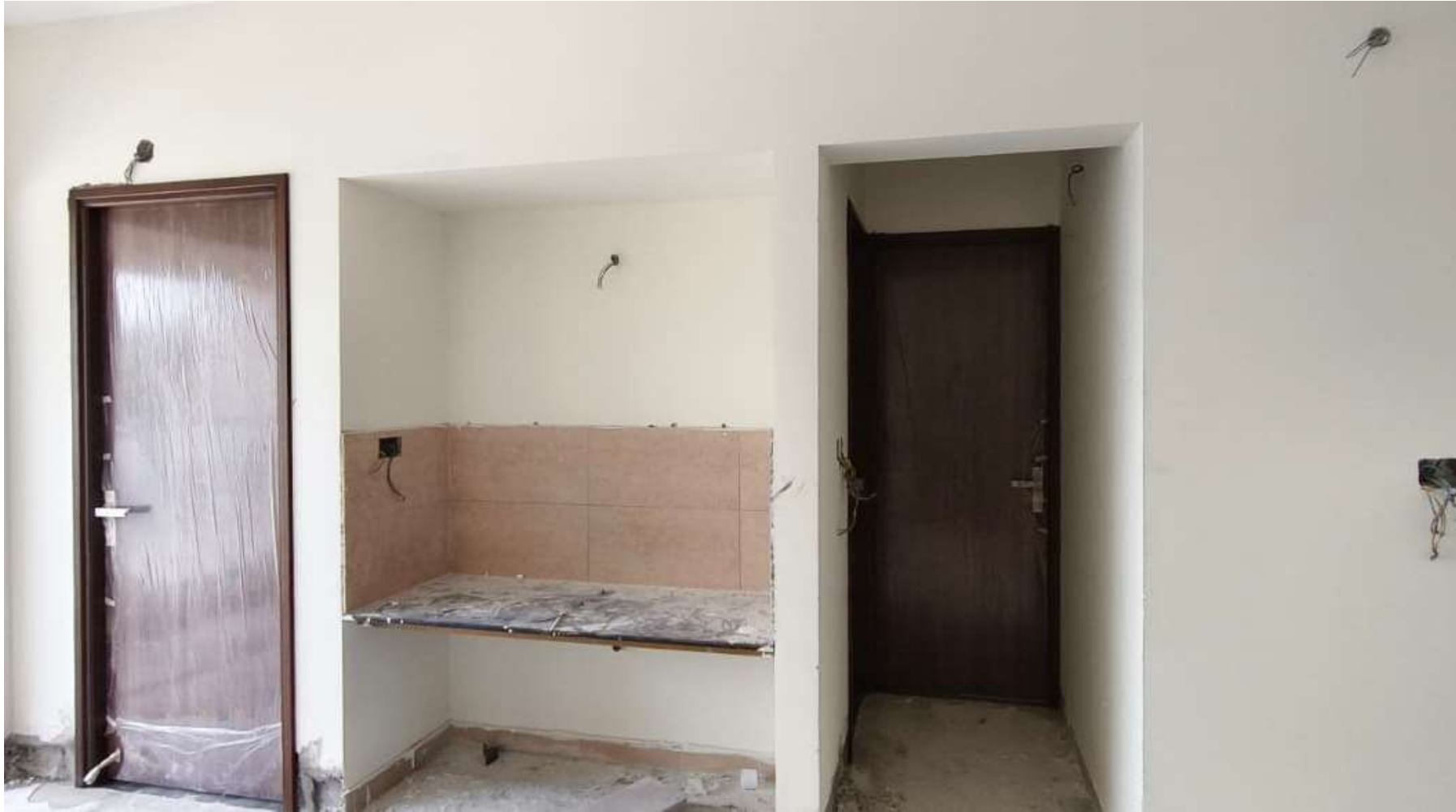
Main Building Pour-2 Up to 2 nd Floor Flat Door Fixing Work Completed.
