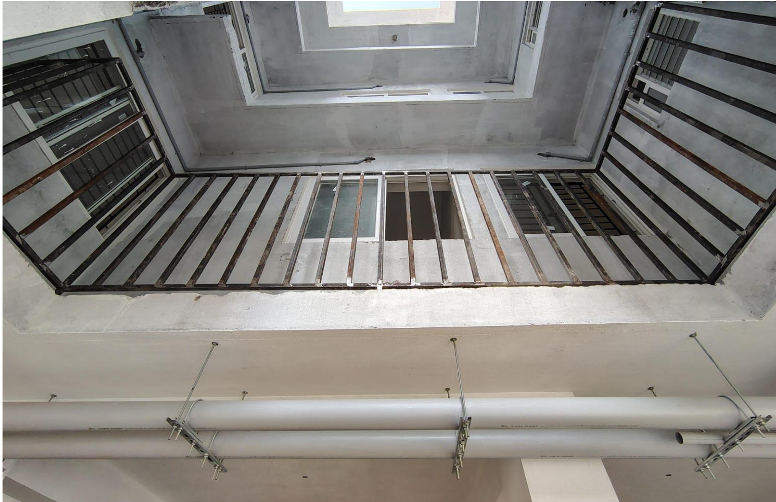
Wing 3D, 3E & 3C – AC Service Slab’s Safety Grill Works in Progress
